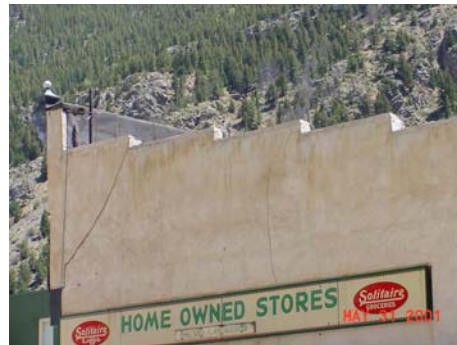
Figure 3. Condition of monitored structures.
